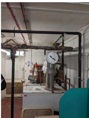
7.5 - Room 5 boiler and door
