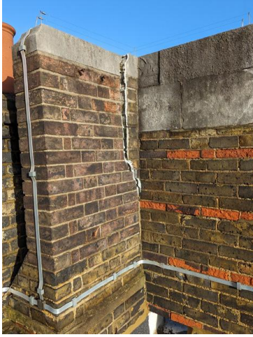
3.9 - Cracked parapet wall
