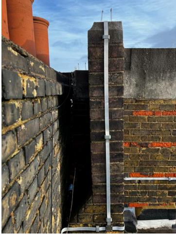
3.8 - Chimney/ parapet gap
