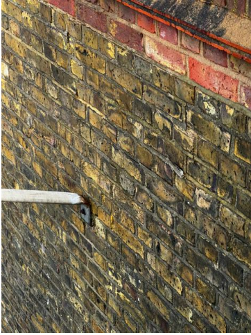
3.7 - Damaged cement fillet
