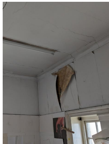
7.69 - Room 36 walls and soffit
