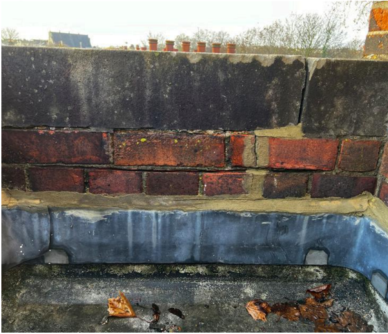
3.13 - Low parapet movement
