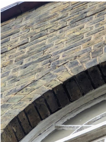
5.3 - NW elevation vertical cracking
