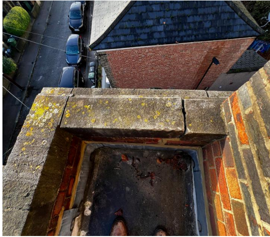
3.14 - Low parapet movement
