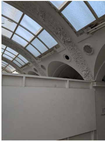
7.59 - Room 34 ventilation grilles
